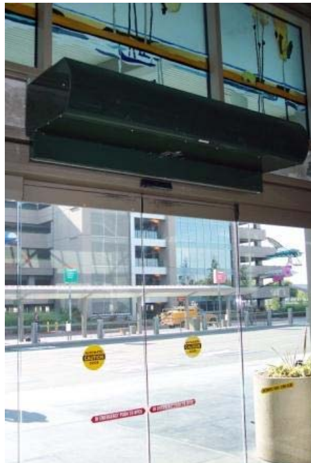
October 17, 2005 - One of the new air curtains at SMF. Photo by Paul Bennett.
